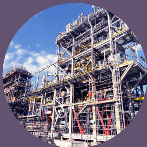
↑ TEG modules 3x300 MMSCFD United Arab Emirates
